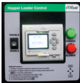
Loading Control: Allen Bradley / Mitsubishi
